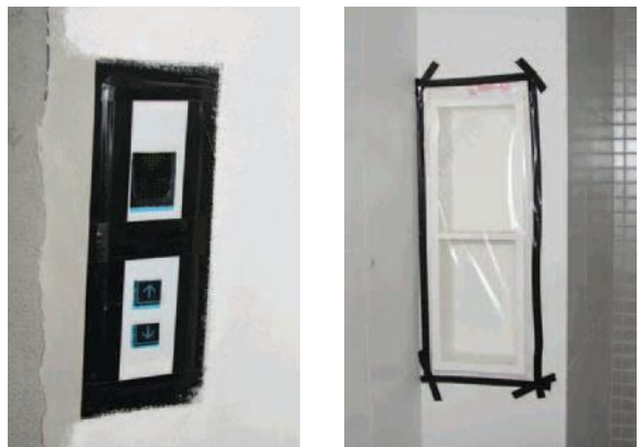
Lift Button Panel and Cabinet
