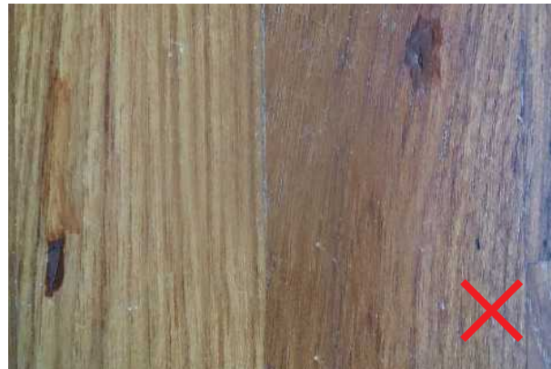
Dents and damages
