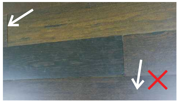
Obvious gaps between engineered wood strips
