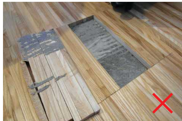
Insufficient adhesive – produces 'cracking' or squeaking sound
